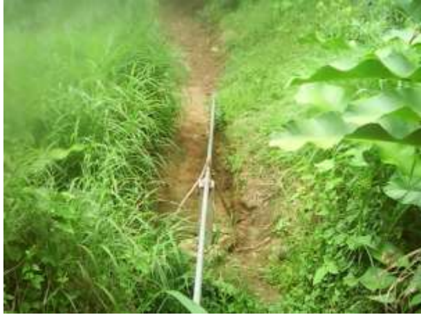
Metal pipe crossing a creek
