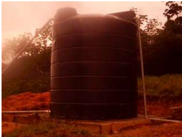
Water tank on the concrete base
